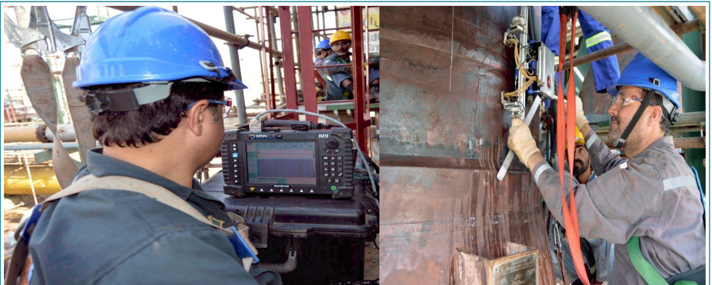
Data Acquisition of Platformer Reactor 301-DN with Motorized WeldRover Scanner by using Time of Flight Diffraction (TOFD) technique at Pakistan Refinery Limited by NCNDT personnel
